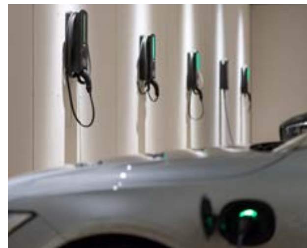
Electric charging stations for clients and employees
