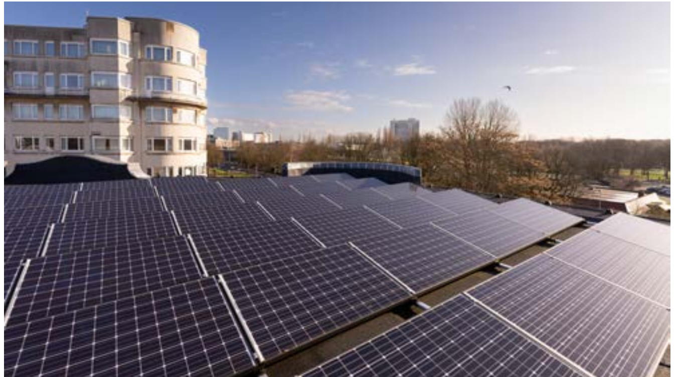
Solar panels on the roof of the head office in Antwerp
